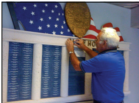
This photograph shows the installer Rick Shapiro, from EDCO making the modifications to the wall.
